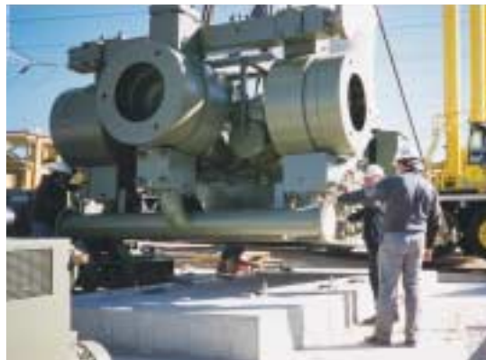
From design and installation, through service, maintenance and upgrade, we are committed to enhance whole life cycle performance to the advantage of existing and new customers.
